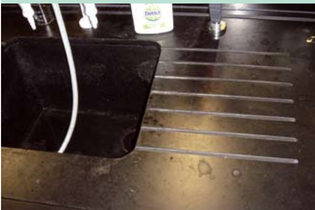
Stains, discolorations and loss of brilliance e.g. on epoxy benchtops
